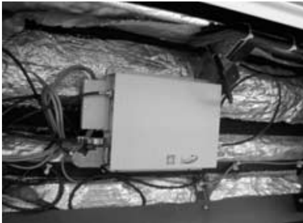
Figure 7. EasyRide reader installed inside a compartment.
